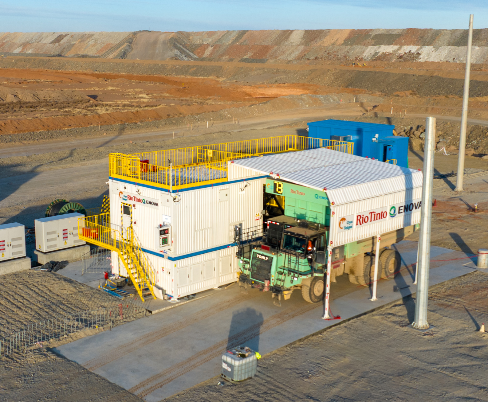
Electric haul truck battery swap station
